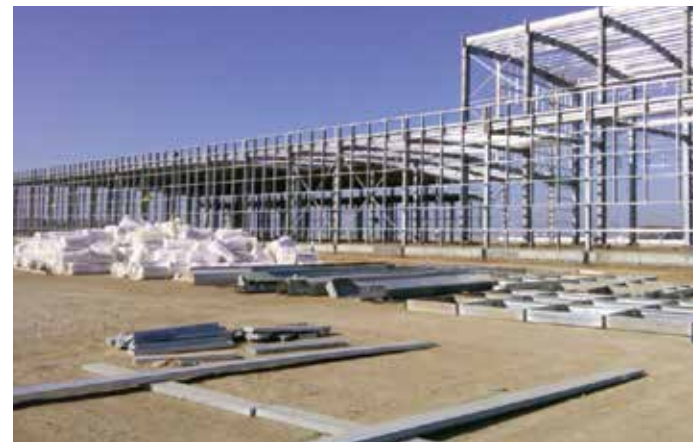
Saudi Arabia Plant Building 5960 m 2
